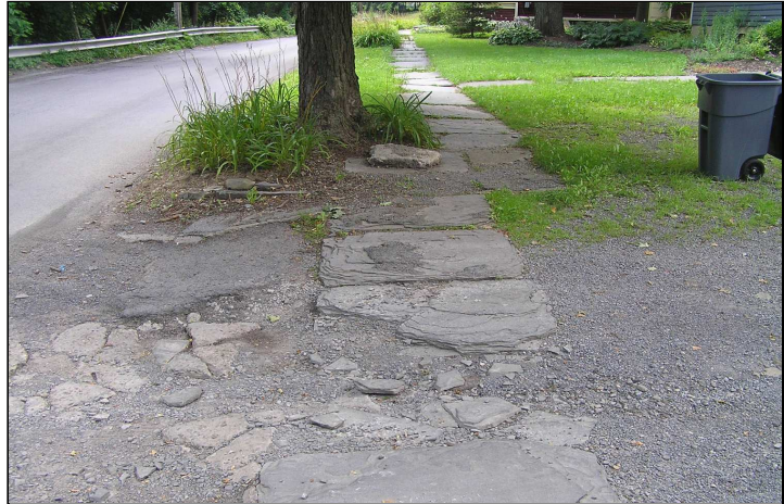
Example of Sidewalk in Deteriorated Condition
