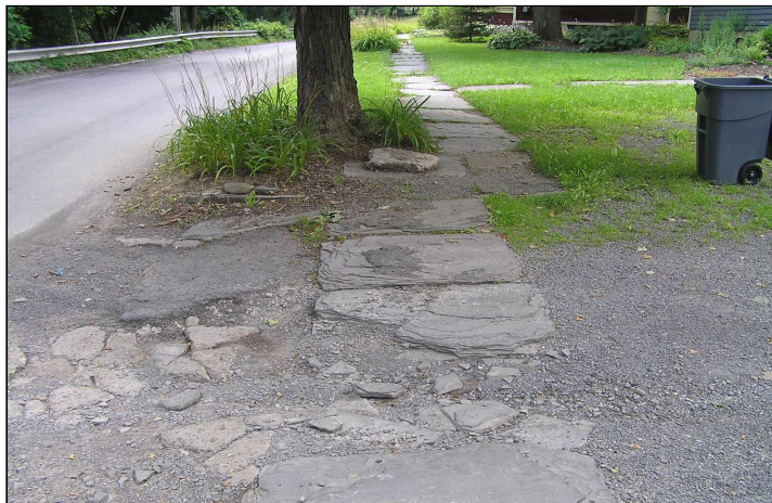
Example of Sidewalk in Deteriorated Condition
