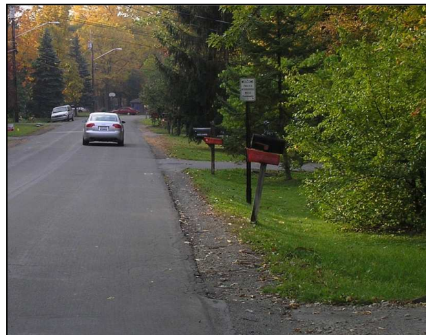
Washed Out Shoulder Along Collector Road In Northeast Ithaca
