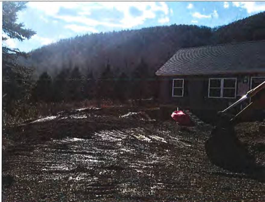
Site visit to 111 Patchen Court 2/27/18 showing partially built home and extent of disturbed soil.
