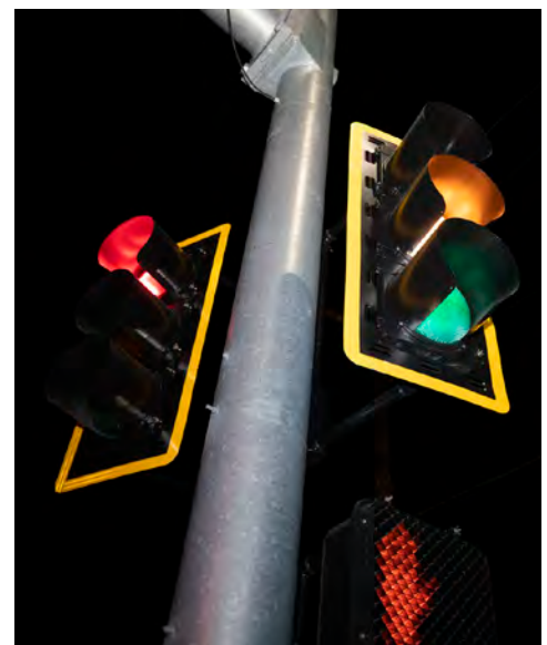
Signal Backplate (Source: Nevada DOT)
