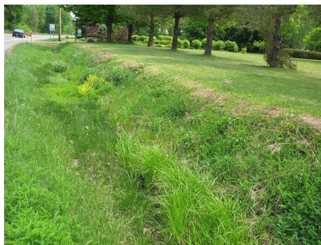
Roadside ditches in the Etna area are a major contributor to sediment in Fall Creek.
