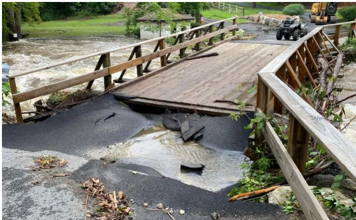
Damage to bridge
