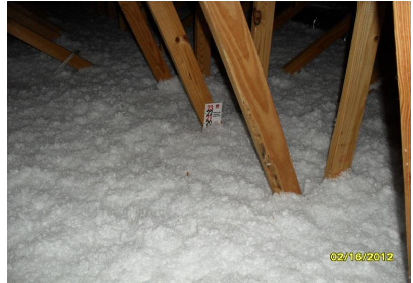
Nice R-50+ Attic Insulation
