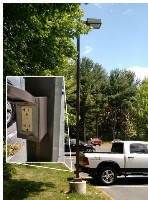
Figure 20: Outlets Available for Charging at Cornell Business Park
